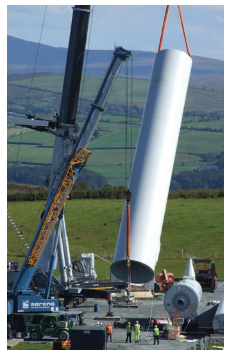
A crane lifts a section of the base tower for erection on the controlled hard standing area at Carrickatane wind farm. With so many contractors on site during the turbine erection phase, safety coordination is a key issue.
