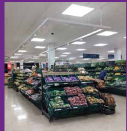
ESB Smart Energy Services LED lighting project at a Tesco store.
