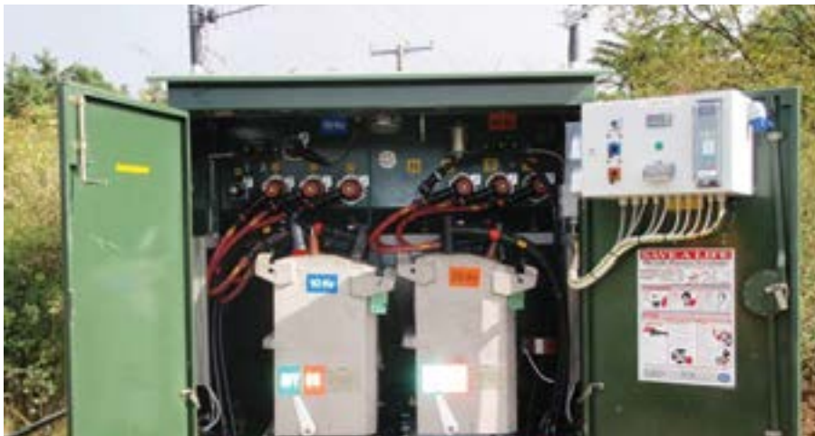
Interface Transformer (IFT) used to step up voltage from 10kV -20kV
