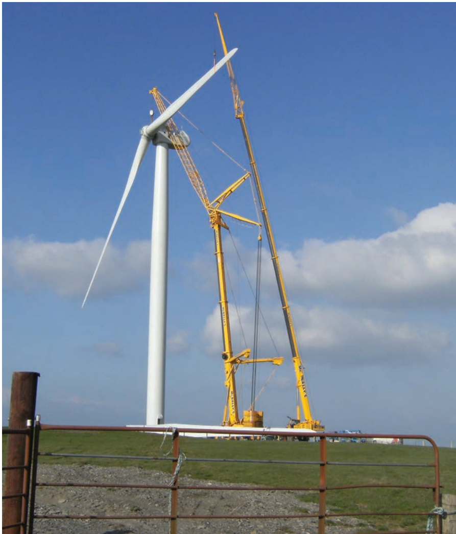
Turbine erection on a wind farm is a high risk activity during the construction process that requires competent contractors and coordination of activity.
