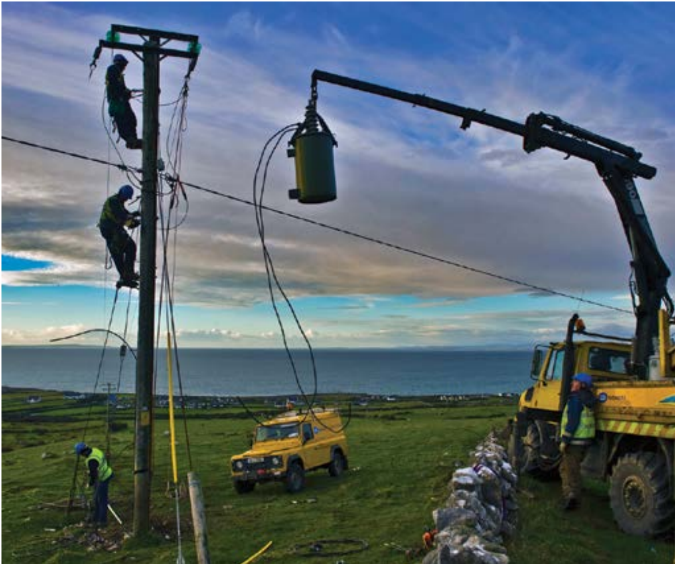
Upgrading of rural distribution network from 10kV to 20kV delivers a higher quality supply to the periphery of the network.
