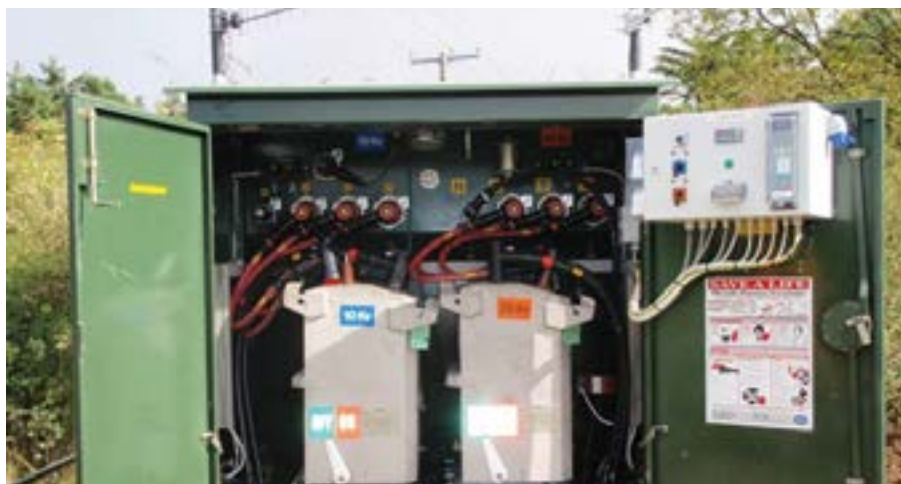
Interface Transformer (IFT) used to step up voltage from 10kV -20kV
