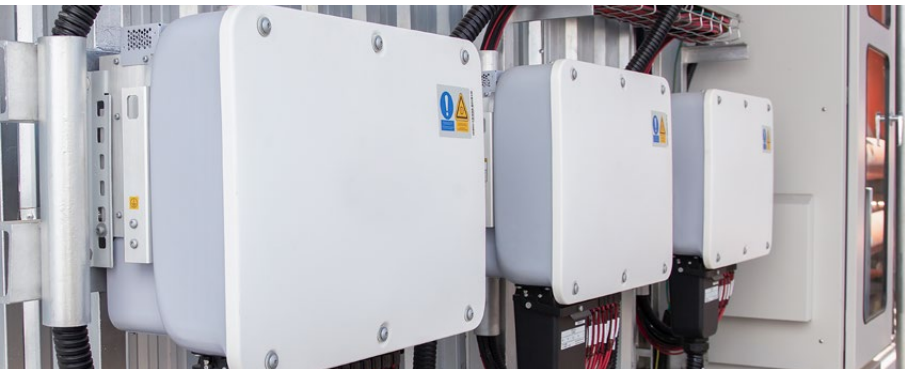
Inverter of solar cell power generation system
