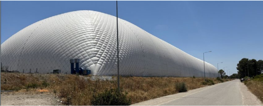
CO 2 battery storage (Credit: Energy Dome)
