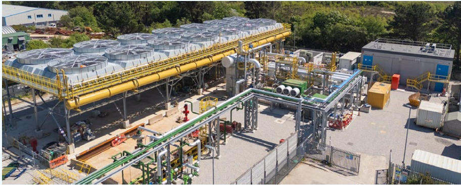
GEL's 3MW United Downs EGS project in Cornwall showing the two wells, ORC heat exchangers, turbine and generator (Credit: Geothermal Engineering LTD)
