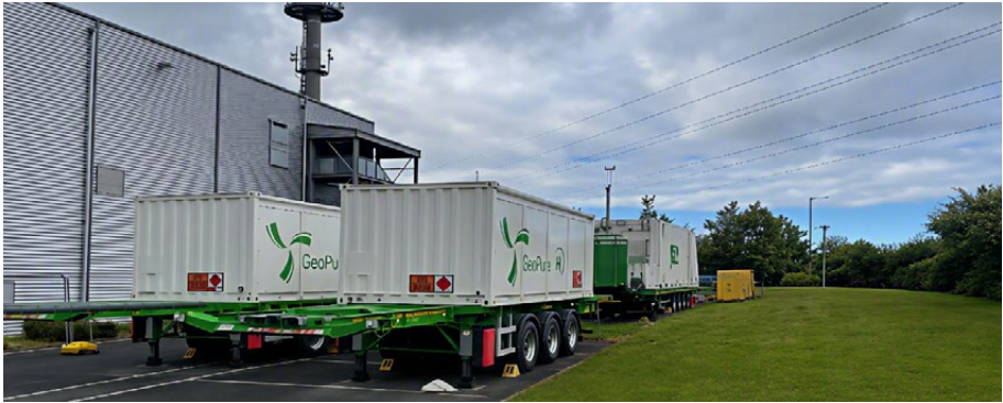
ESB's hydrogen fuel cell generating electricity for a data centre in Dublin
