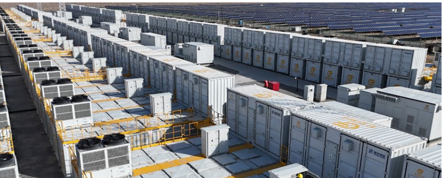
Flow Battery Storage (Credit: © Rongke Power (RKP))
