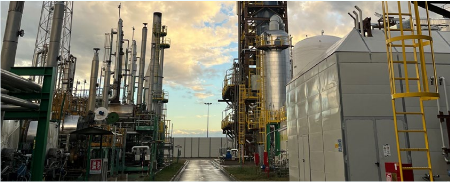
The Ravenna Carbon Capture and Storage (CCS) plant located on Italy's east coast.
