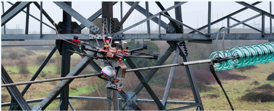
ESB Networks drones placing DLR sensors on power lines
