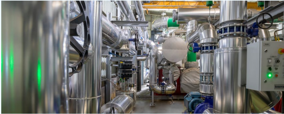
Industrial heat pump system (Credit: Turboden Sp.A, a Group Company of Mitsubishi Heavy Industries)
