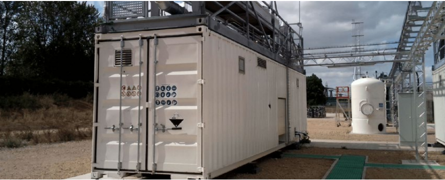
A photo of ESB's first electrolyser – it has been fabricated and will be installed in Aghada Power Station in 2027
