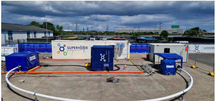
Superconductor demonstration project, Blyth, UK (Credit: SuperNode)
