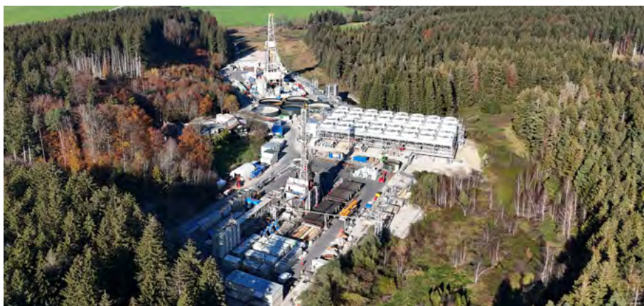
Eavor project in Geretsried, Germany (Credit: Eavor)
