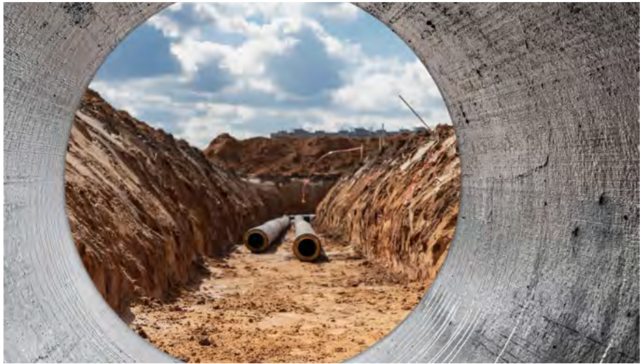
District Heating Pipes
