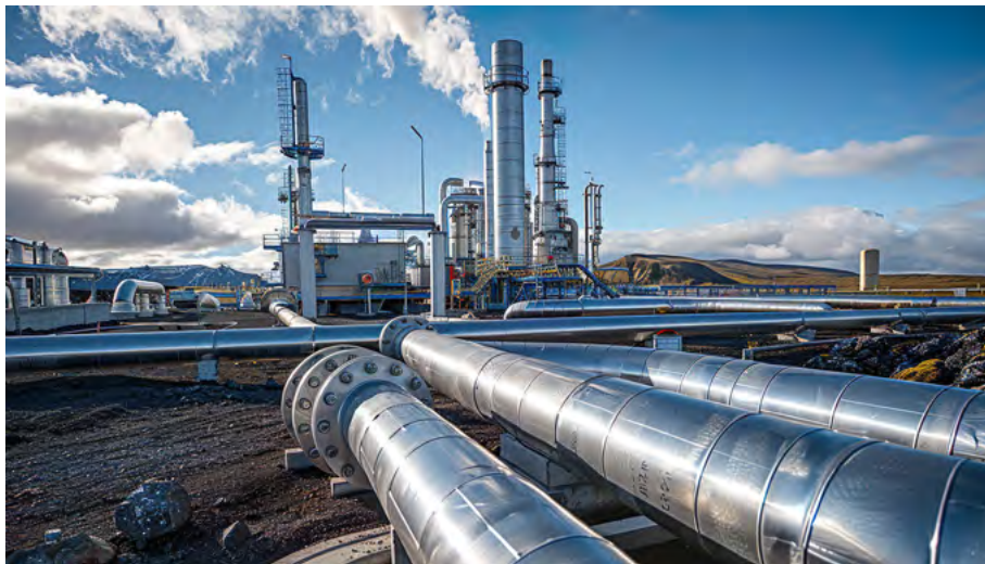
Carbfix project in Iceland
