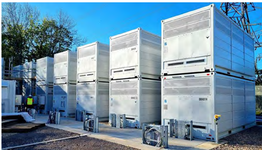
Vanadium Flow Batteries in Oxford, UK. Credit: Invinity
