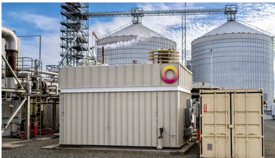
Rondo Brick Storage California, Credit: Rondo
