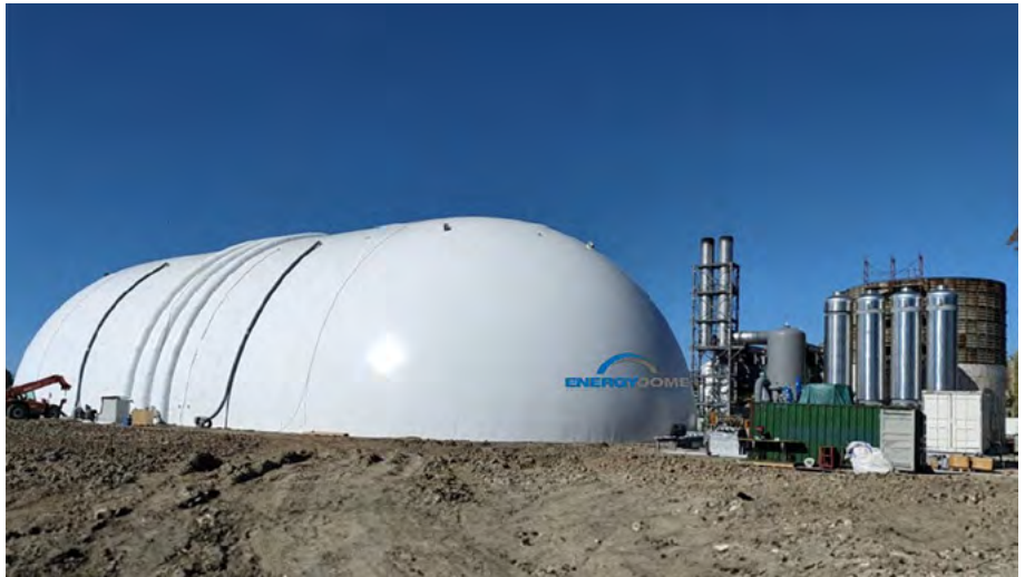
Energy Dome CO 2 battery, Sardinia, Credit: Energy Dome
