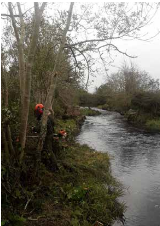
Selective clearance of bankside vegetation at 'Divers Pool', on the Clady River.
