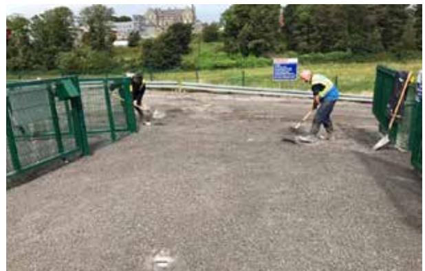
The entrance to the Erne Eel release site on the Lower Erne system being improved.
