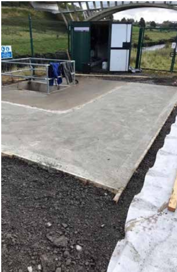
The same site with the area being prepared for concrete being laid.
