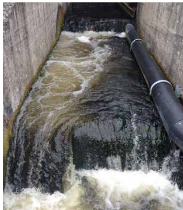
A view of the Parteen Weir fish pass.
