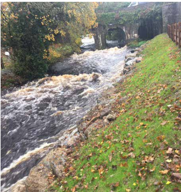
The Woodford River in high flows with a series of instream stone weirs and rock armor along the near side of the riverbank.
