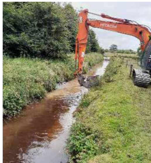
Before, after work photographs taken on the thalweg below Cloonard Bridge (Upper Francis River).
