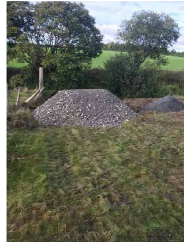
Stone fill being used for the creation of a livestock drinking area.
