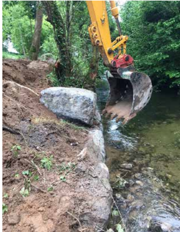
A short section of rack armour being built on the Ballyfinboy River.
