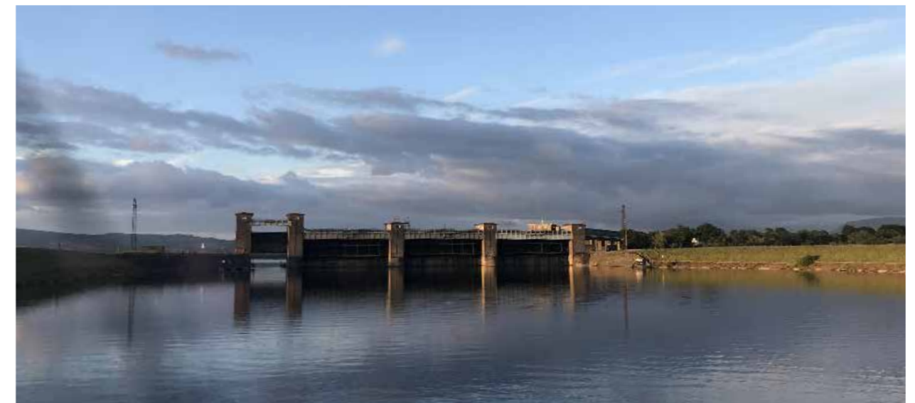
The regulating gates at the entry point to the Ardnacrusha headrace canal.
