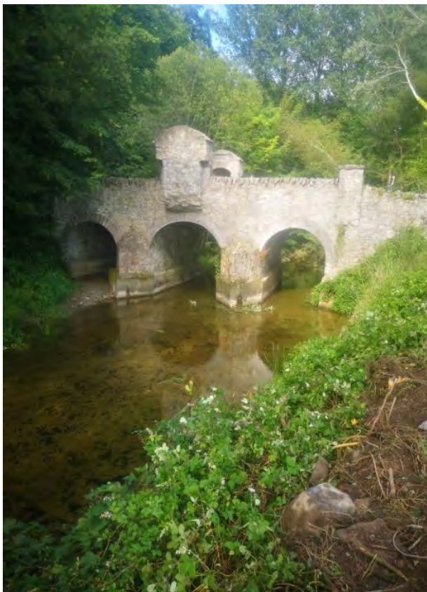
An area of the Ballyfinfinboy River where bank slippage has occurred. The large limestone boulders have been delivered to the site and aligned along the riverbank. A tracked machine will selectively place these along the riverbank to prevent further slippage.
