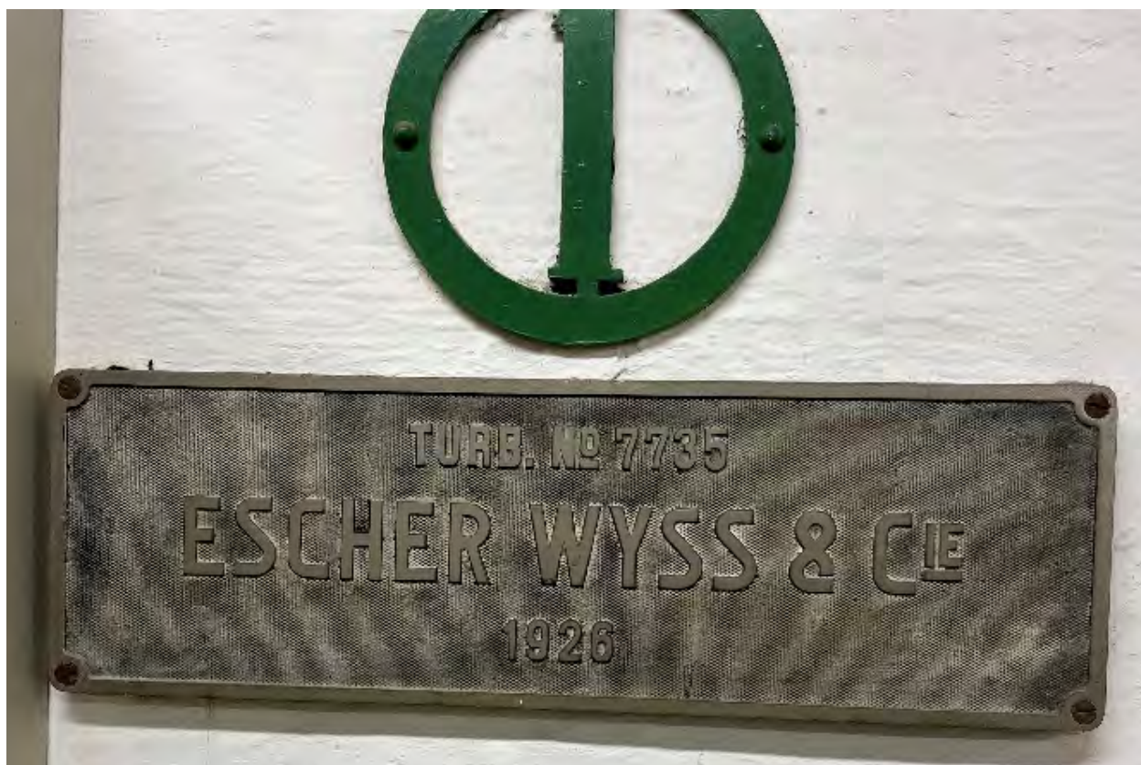
A view of one of the generators at Ardnacrusha station.
