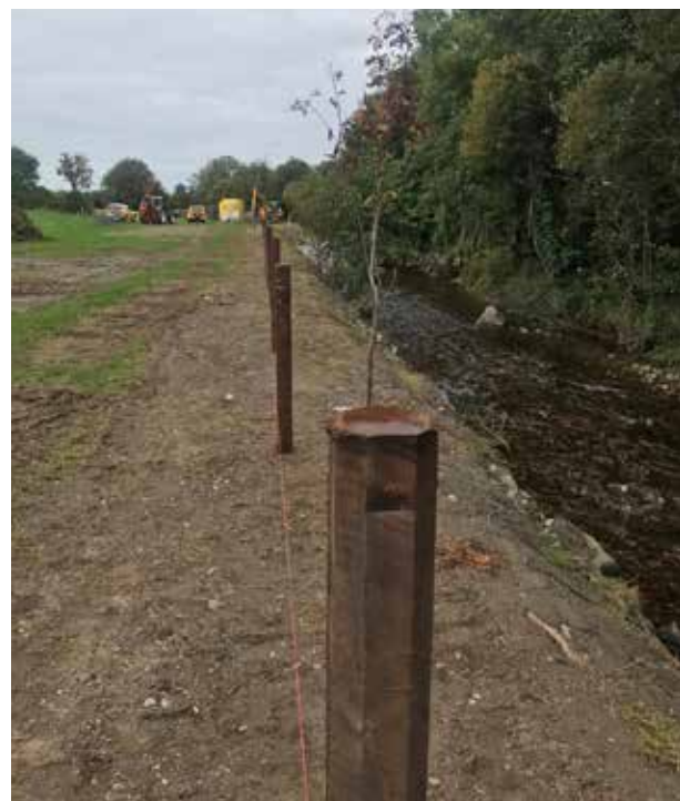
New fencing being erected along a newly rock armoured section of riverbank on the Breaghmore site on the Camcor River. Random boulders have also been placed within the pool area above the newly constructed stone vortex weir.
