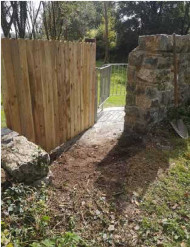
A newly erected public access point on the banks of the Ballyfinboy River.
