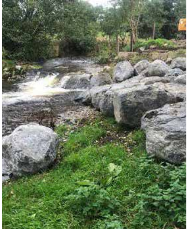
Construction of a stone vortex weir and bankside rock armour on the Breaghmore section of the Camcor River.
