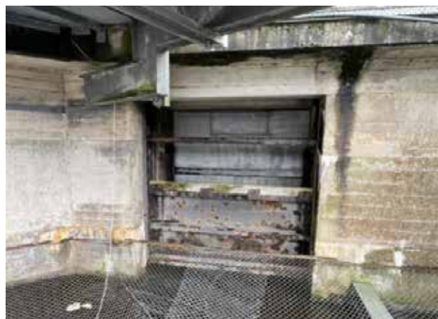
The presently closed Erne stations smolt gates, which will be fitted with a movable flume gate over which water will be spilled to provide an alternate downstream route for migrating fish.
