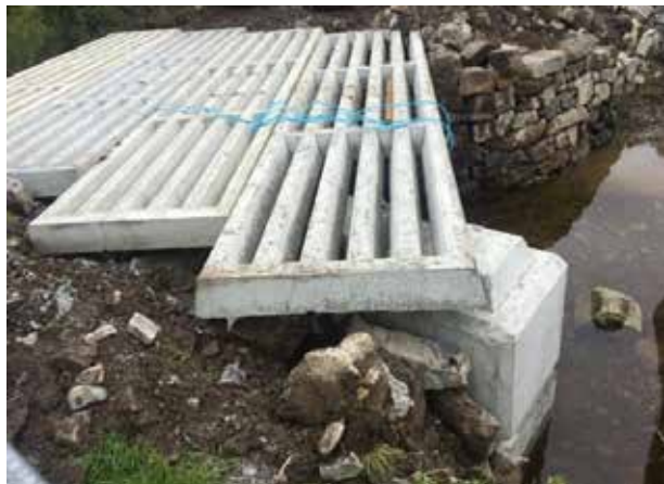
Cattle slats being lifted into place and concrete being poured to form a bridge.
