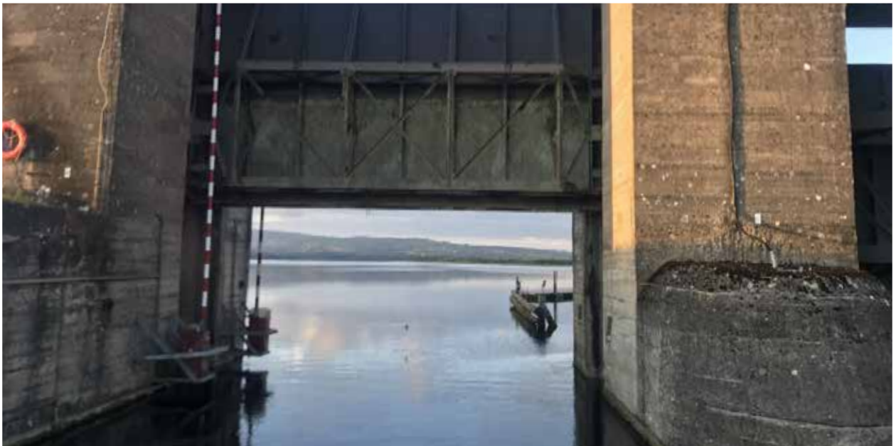
The navigation gate at the entry point from the Ardnacrusha headrace canal into Parteen regulating Weir.
