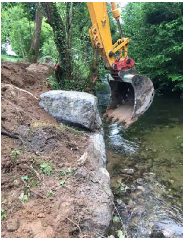
A short section of rock armour being built on the Ballyfinboy River.
