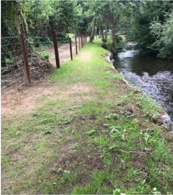
Rock armour along a short section of riverbank and new fencing erected.
