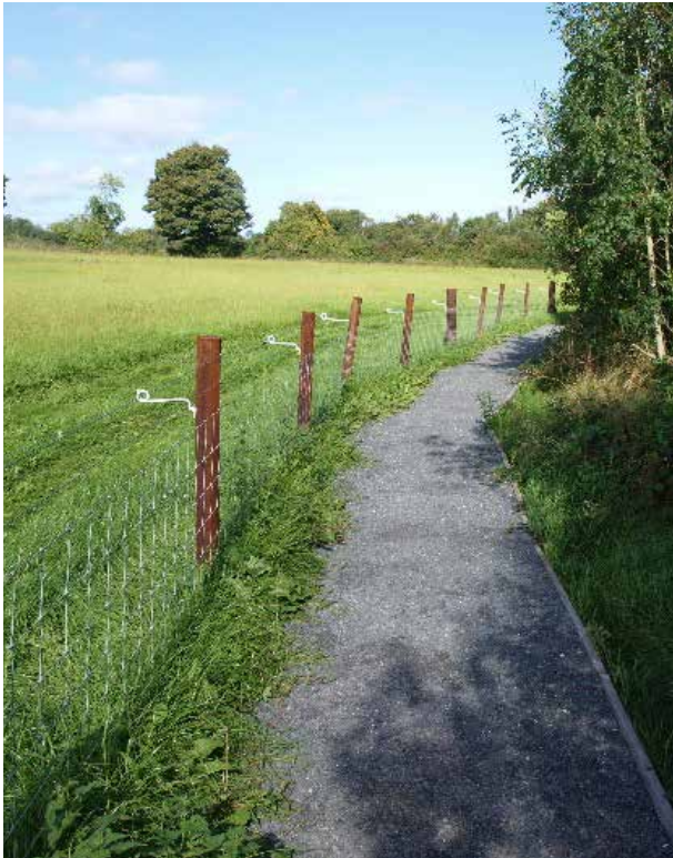
A fenced footpath area leading to the new bridge over 'Conway's Canal' in Castleconnell.
