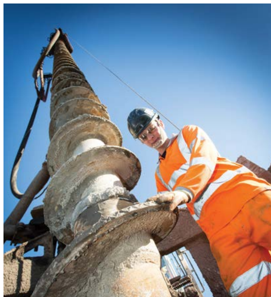
As of January 2014, the numbers of workers on site has increased to over 400 people.
