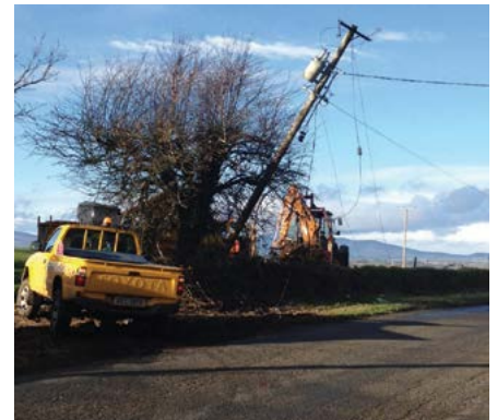
ESB Networks at a location in Enniscorthy where severe damage was caused.
