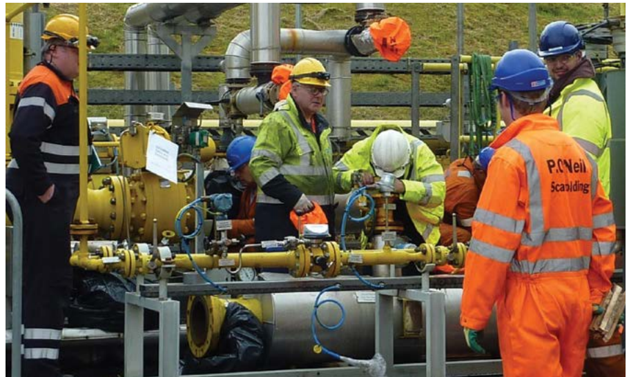
Jon Taggart and Derek Gallagher, both Coolkeeragh ESB with various contractors during the Fuel Gas Heat Exchanger Inspection.
