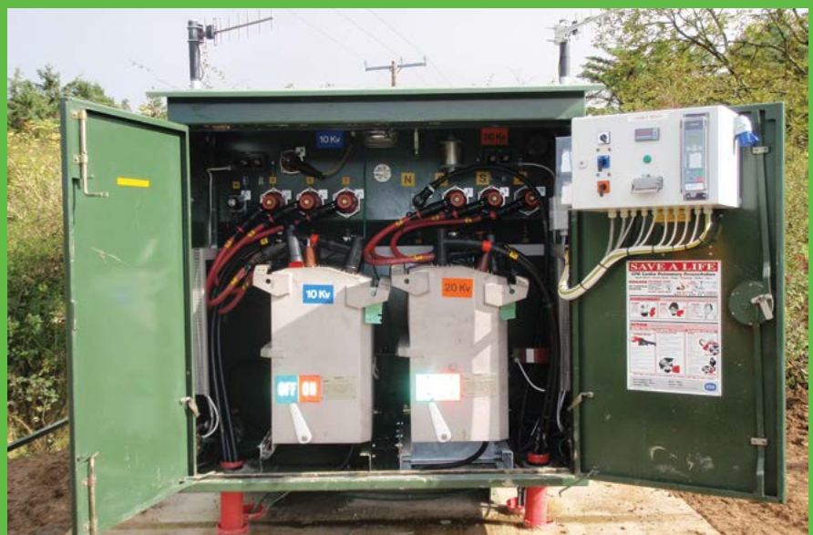
A retrofitted transformer cabinet with the additional space for fitting of new protection equipment.
